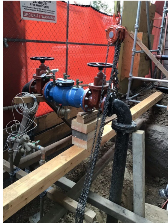
Figure 2 – installed Backflow Preventer
