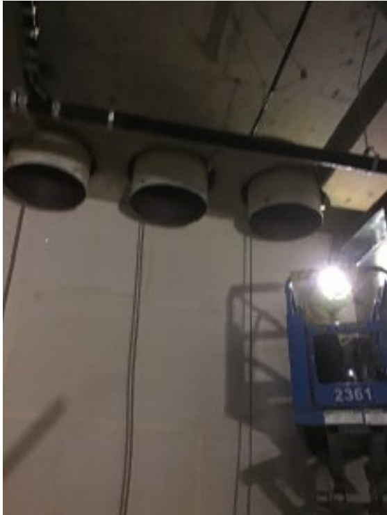
Figure 1 – Level 1 Trash Chutes
